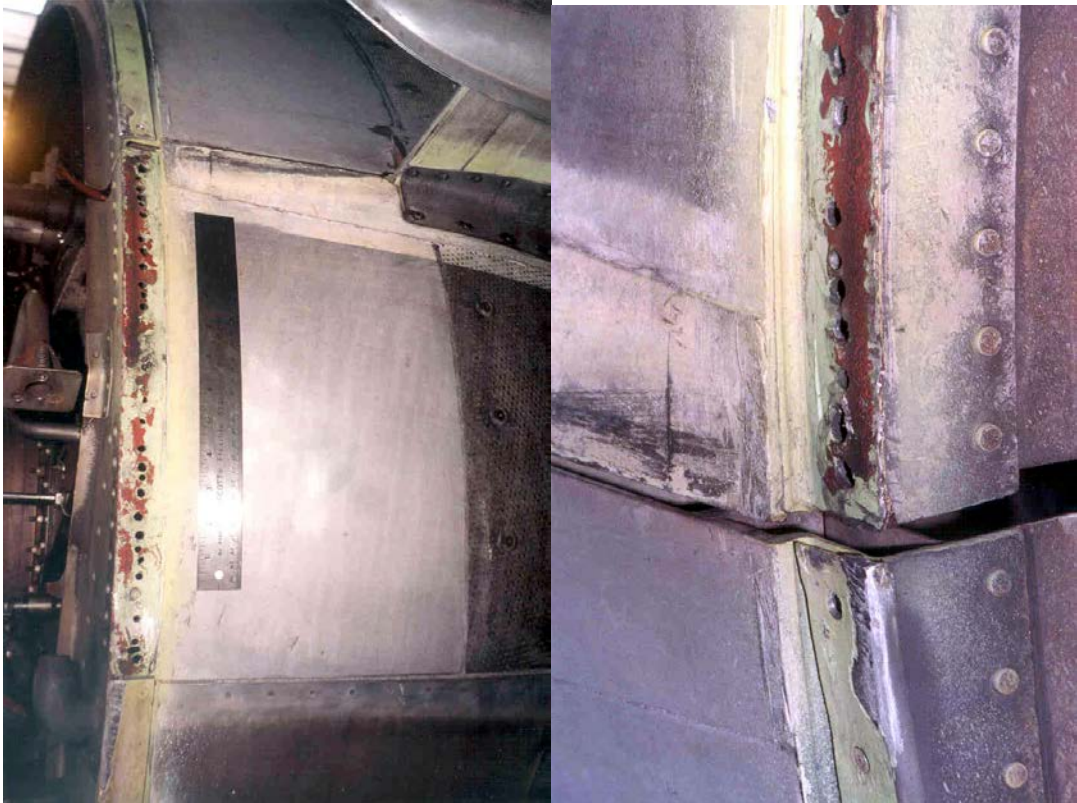
Figure 52: Pictures showing the position of the wear strip
